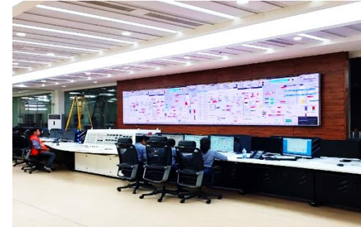
BF Control Room
